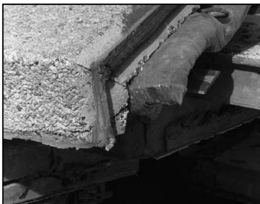
Top: An apartment building from the 1960s being recycled. Middle and bottom: It can be deconstructed - but a closer look shows that the sealants contains large amounts of PCB which makes it difficult and expensive to reuse the components
