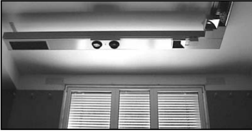
New artificial lighting system
