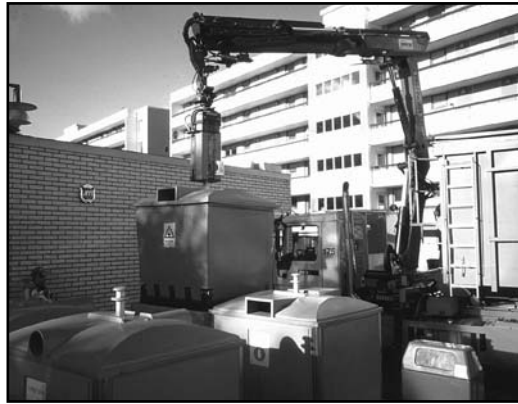
A well planned building site will make the recycling and sorting of waste easy
