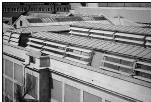
Automatic light control louvres on gallery roof
