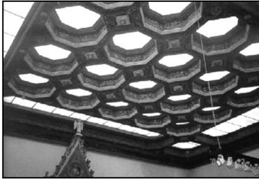
Bardini Museum: Existing wooden / glazed ceiling
