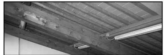
The renovated ceiling of Bardini Museum is constructed using traditional techniques and materials
